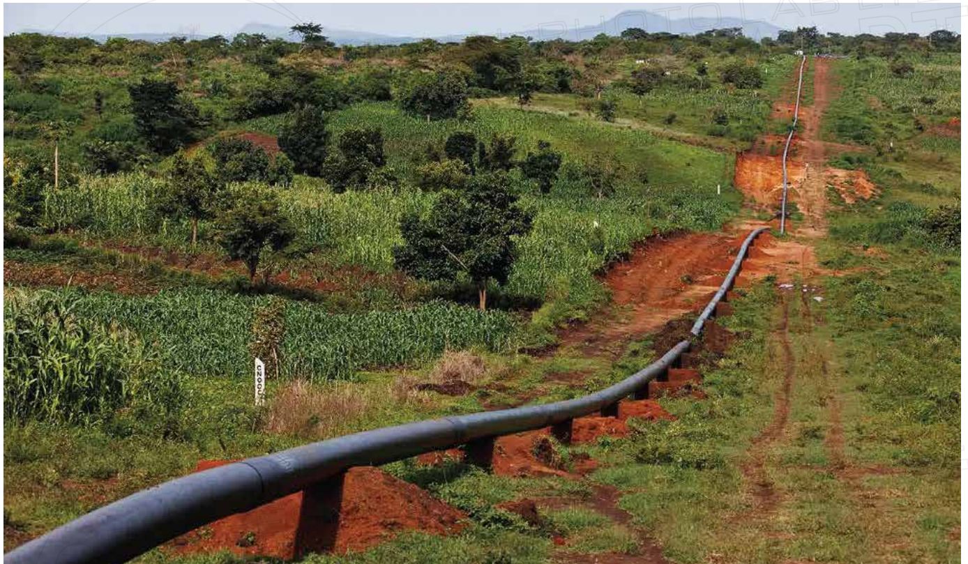
Section of East Africa Crude Oil Pipeline: “Local firms often compete against better-resourced international contractors, particularly on high-value or complex projects.” Photo https://www.thehabarinetwork.com/east-african-crude-oil-pipeline-expected-to-yield-significant-benefits-to-region
